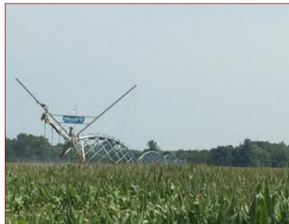
Leachate distribution system.
